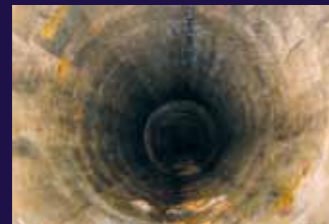
DN150 DRINKING WATER LINE
