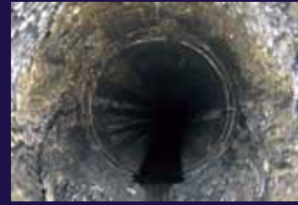
DN250 SLUDGE WATER LINE
