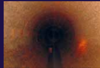
DN300 WATER TREATMENT PLANT
