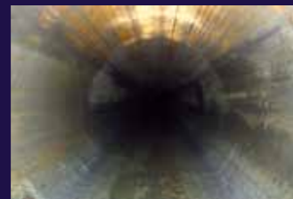
DN200 WATER COOLING LINE
