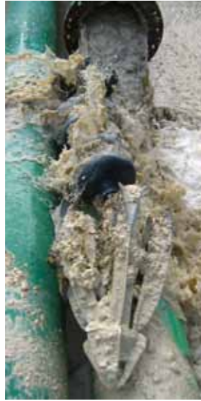
16" LATEX PRODUCTION PIPELINE
